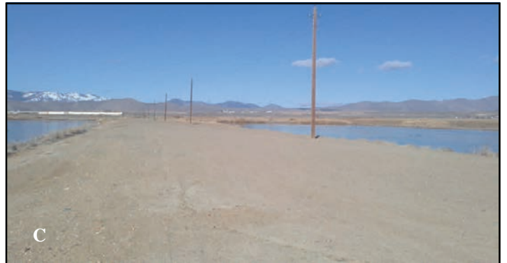
Figure 1. Large source reduction project at the Lemmon Valley sewage treatment facility before (A), during (B) and after completion (C).
