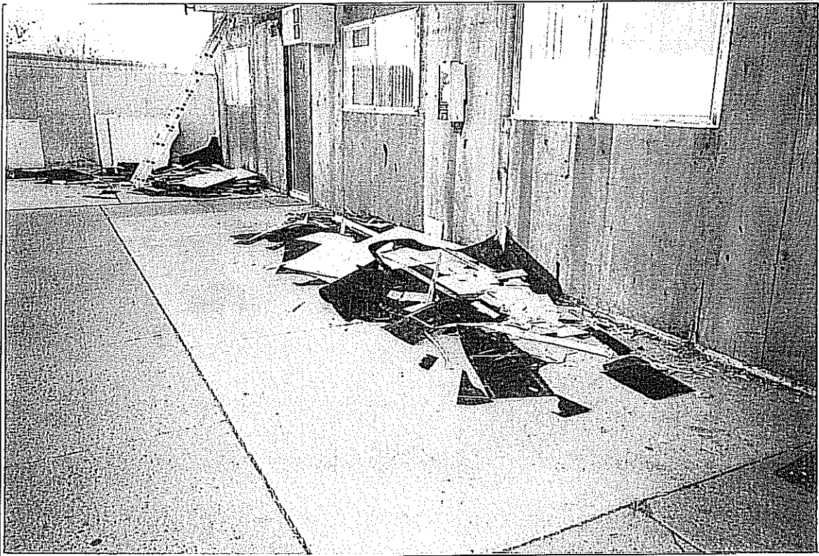
Photographs #3-#4 depict improper work practices for handling asbestos-containing transite siding.
